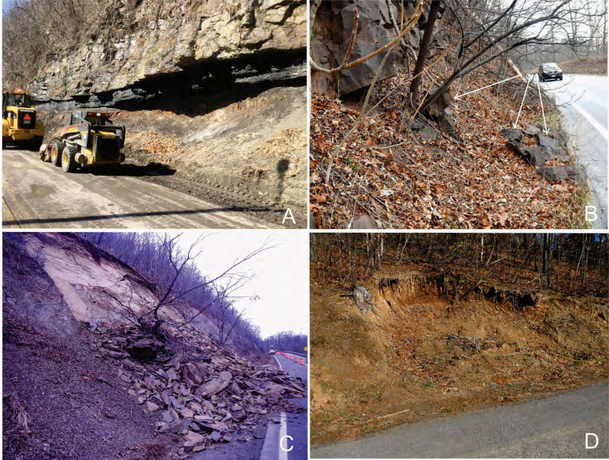
Figure 14. Type of slope failures and resulting hazards identified during this study. A, Rockfall. B, Rock roll. C, Rockslide. D, Slump (rotation) scar.
