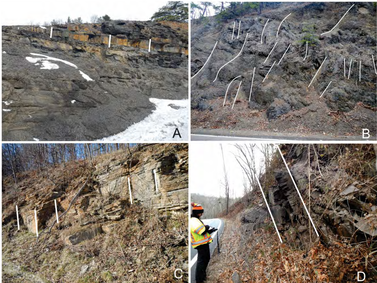
Figure 15. Failure plane character. A, Discontinuous and favorable orientation. B, Discontinuous and random orientation. C, Discontinuous and adverse orientation. D, Continuous and adverse orientation.
