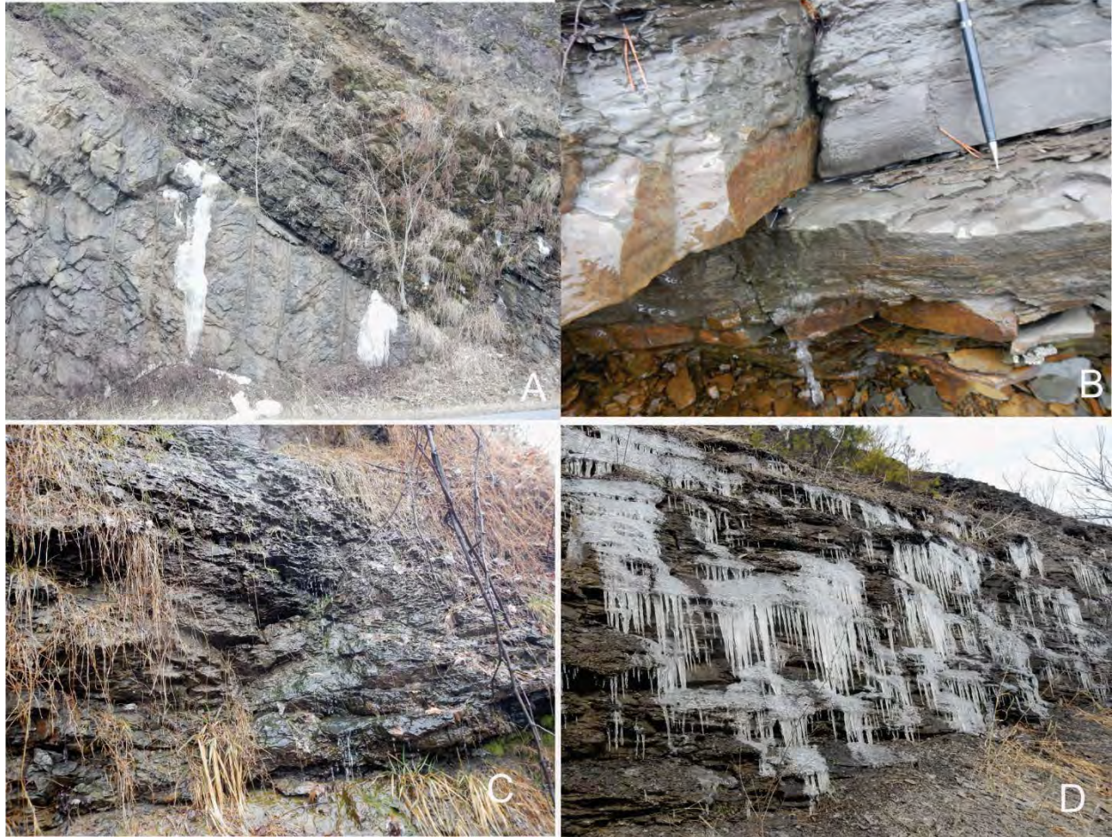
Figure 11. Degrees of variation in the amount and distribution of water on roadside slopes. A, Water seeps along stratification. B, Water seeping along joints and fractures. C, D, Water covering the surface of outcrops.
